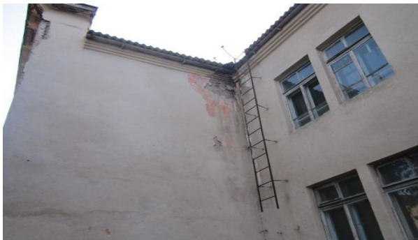
Figure 5 and 6. The deteriorating state of School #44 in Bishkek
